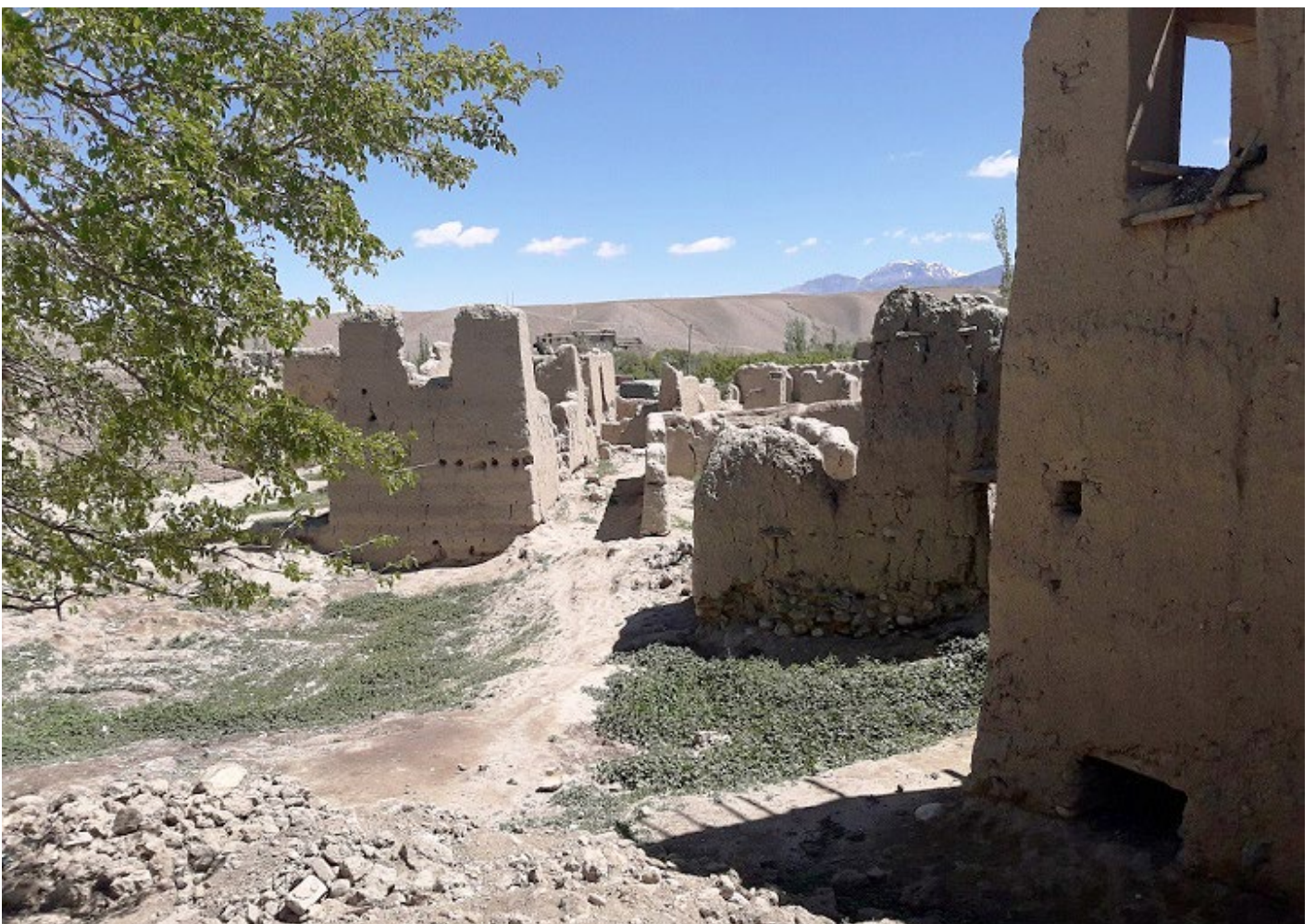
Shelter needs are high in Logar, where 649 IDPs and returnees live in tents or open air and 16% of all houses are either severely damaged or completely destroyed, like these houses in Khoshi district. © IOM 2020
