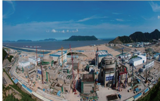
An Overall View of Taishan NPP
