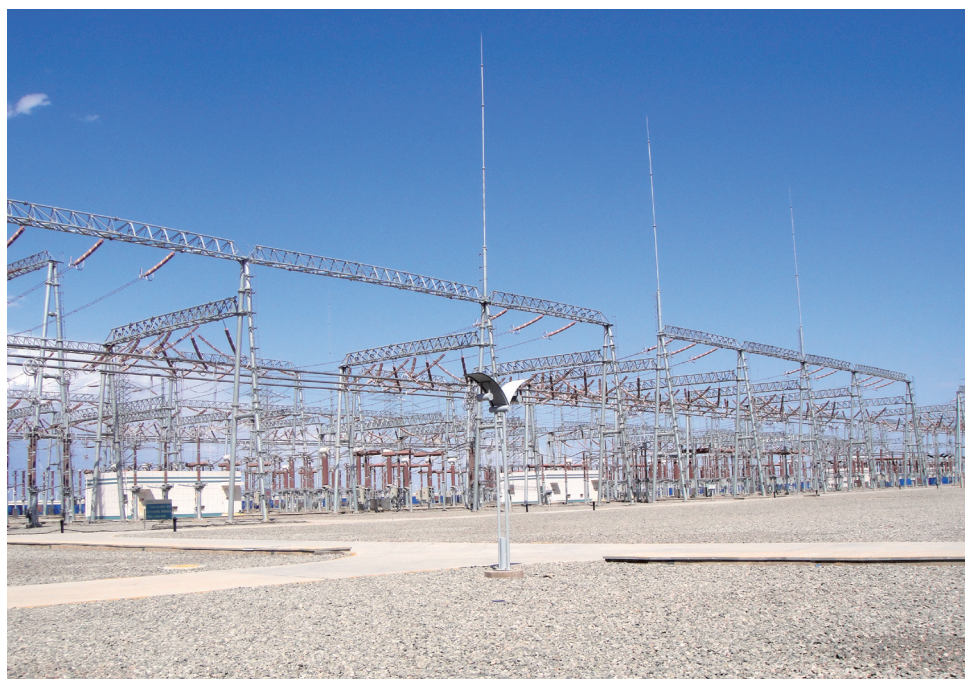
Electric Power Transmission and Distribution Project of the 750kV Channel II Interconnection between Xinjiang and the Northwest Power Grid Main Network
