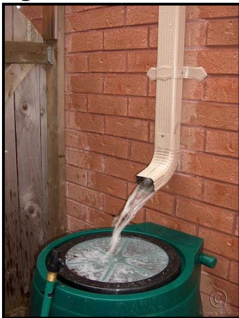
Figure. 4 Rainwater collection (through downpipes and sieves)
