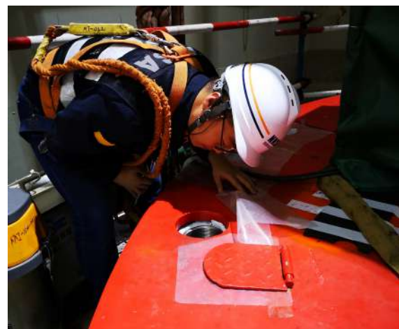
Figure 16. Onsite inspection of steam generator bolt holes of HTGR Demonstration Project by inspectors
