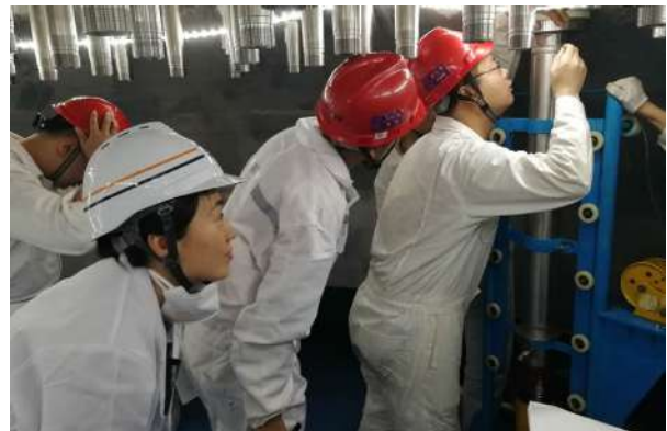
Figure 6. Inspectors conduct the penetration inspection after the hydrostatic test of control rod-driven mechanism seal welding of Hongyanhe NPP Unit 5
