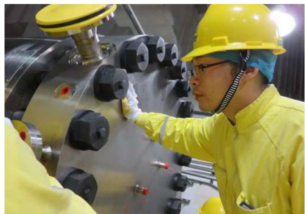
Figure 13. On-site unpacking supervision of newly imported main pumps by inspectors in the radiation control area of Sanmen NPP Unit 2
