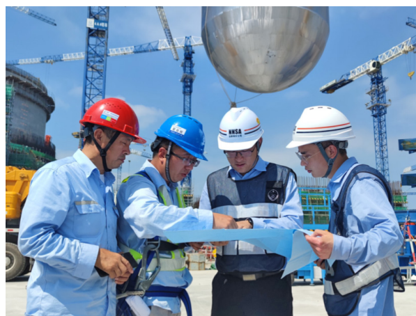
Figure 15. Inspectors Performing Regulatory Inspection for the Reactor Pressure Vessel Installation of Zhangzhou Unit 1
