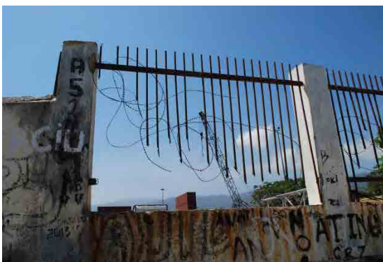
Figure 1.6-11 West Fence (Eroded Area)
