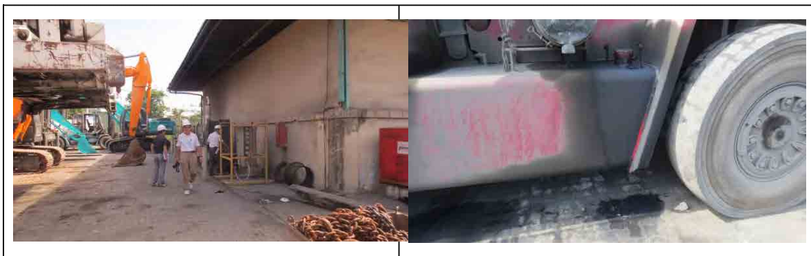
Figure 1.5-5 Oil Leak and Contamination in Workshop
