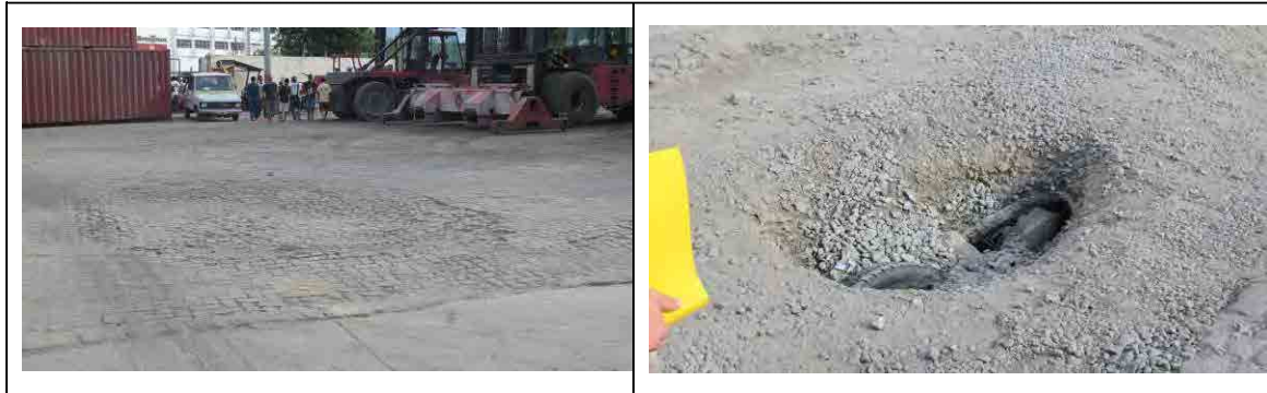
Figure 1.2-5 Deterioration Area of Pavement and Cave-in Point
