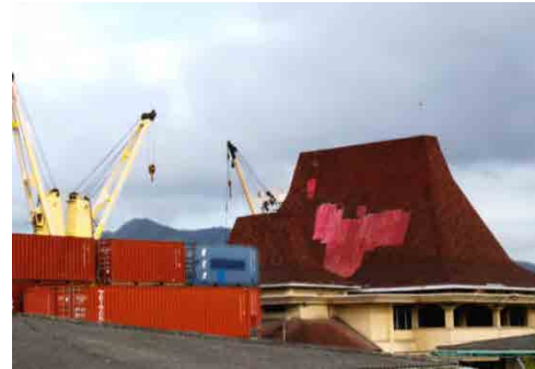
Figure 8.2-4 Badly Damaged Passenger Terminal Building (under repair)
