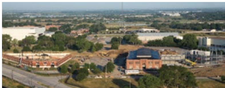
Top: Panorama of Lincoln skyline shows downtown, UNL campus and Nebraska Innovation Campus with Phase I construction boxed. Above: Phase I construction in progress
