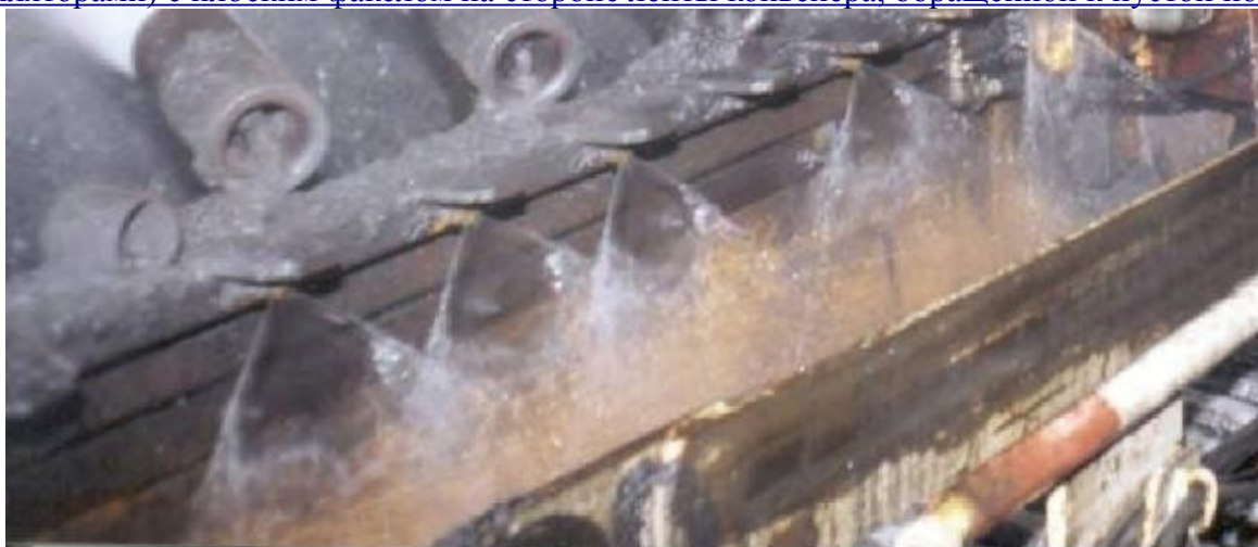
Figure 3-9.—Headgate splitter arm with flat-fan sprays mounted on gob side of belting.
