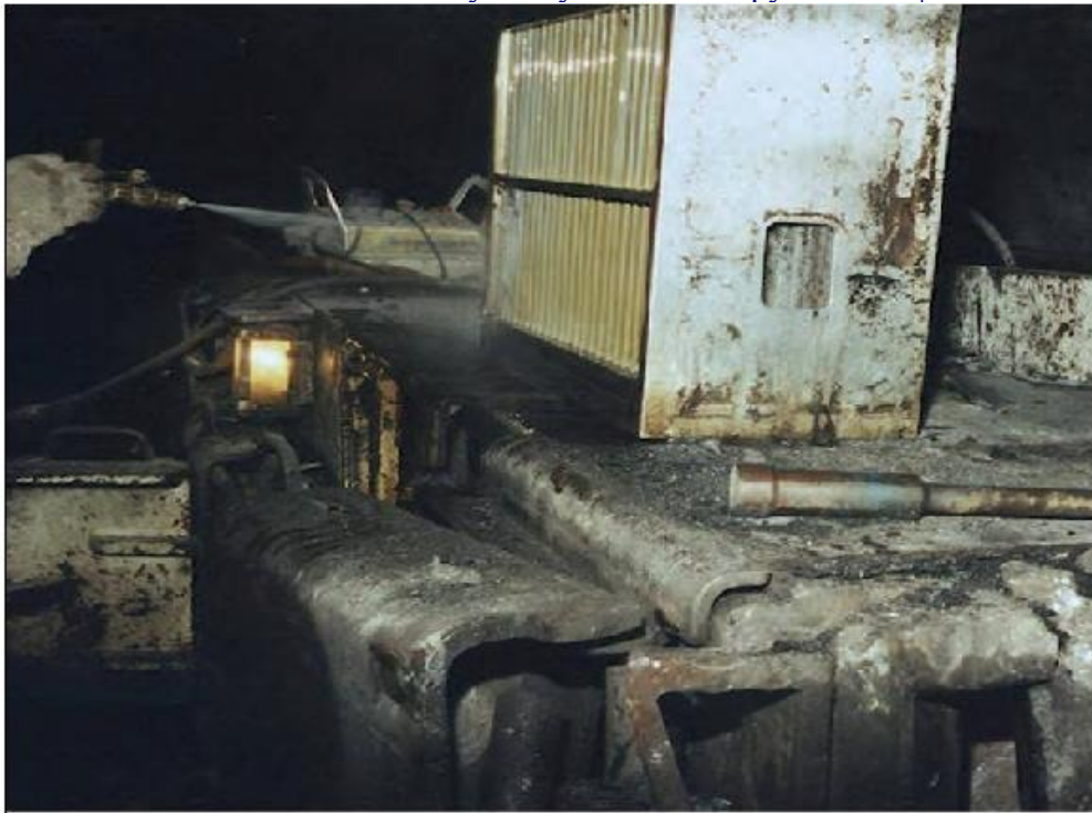
Figure 4-8.—Cleaning the demister with a water nozzle.
