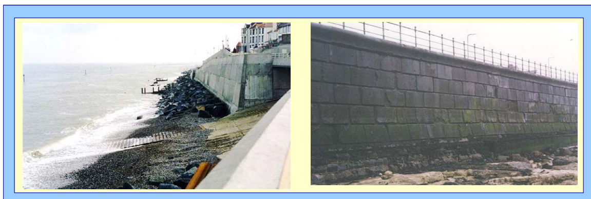
Figure 7.2: Examples of vertical seawalls: (left) modern concrete wall and (right) older stone blockwork wall
