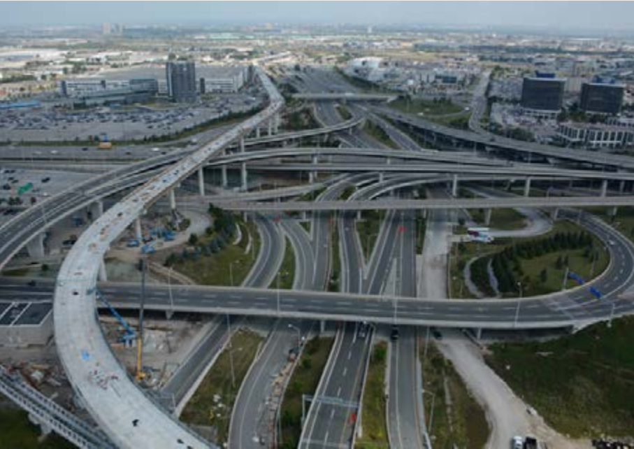
Construction on the Union Pearson Express airport rail link rises above highways.
