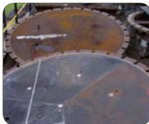
Grade 1.4003/410, Columbus, S. Africa. Carbon steel (top) compared to ferritic (bottom) after 6 years in service.
