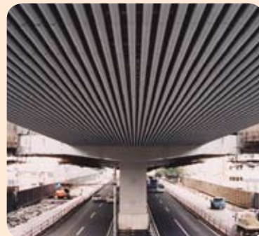
Overpass noise-absorbing plate, Japan.
