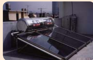
Solar water heater, Taiwan, China.
