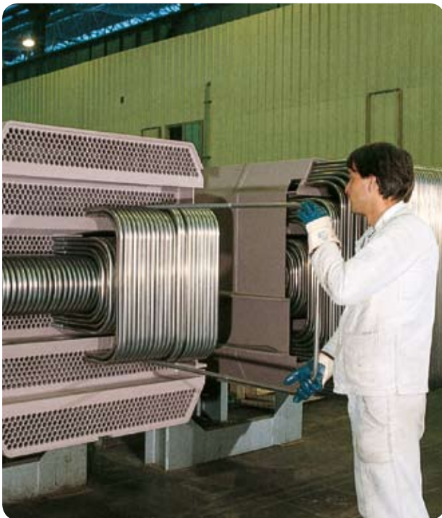
Moisture separator reheater in grade 439, Europe.
