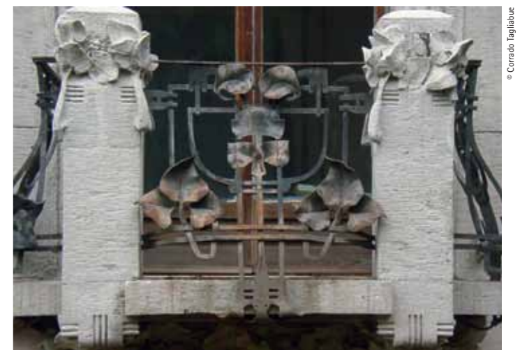
Facade balcony at the first floor level, outstanding for its wrought iron work manufactured by the Mazzucotelli company
