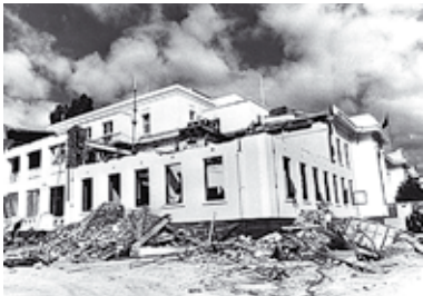
Demolition work in progress as part of the extensions that were carried out in 1972–73. This included the addition of a new Prime Minister's Suite.
