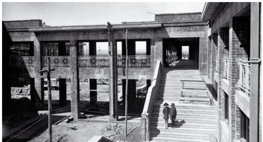
Two young girls stand on courtyard steps of the building during its construction in 1926.
