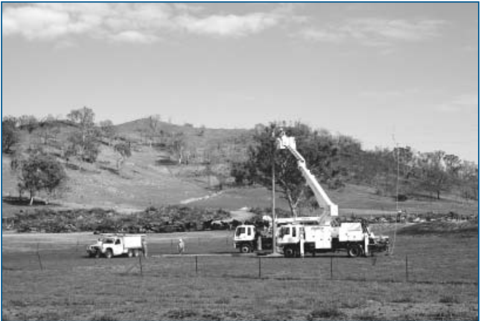
Repairing powerlines as part of the recovery process. Photo courtesy ACT Publishing Services.
