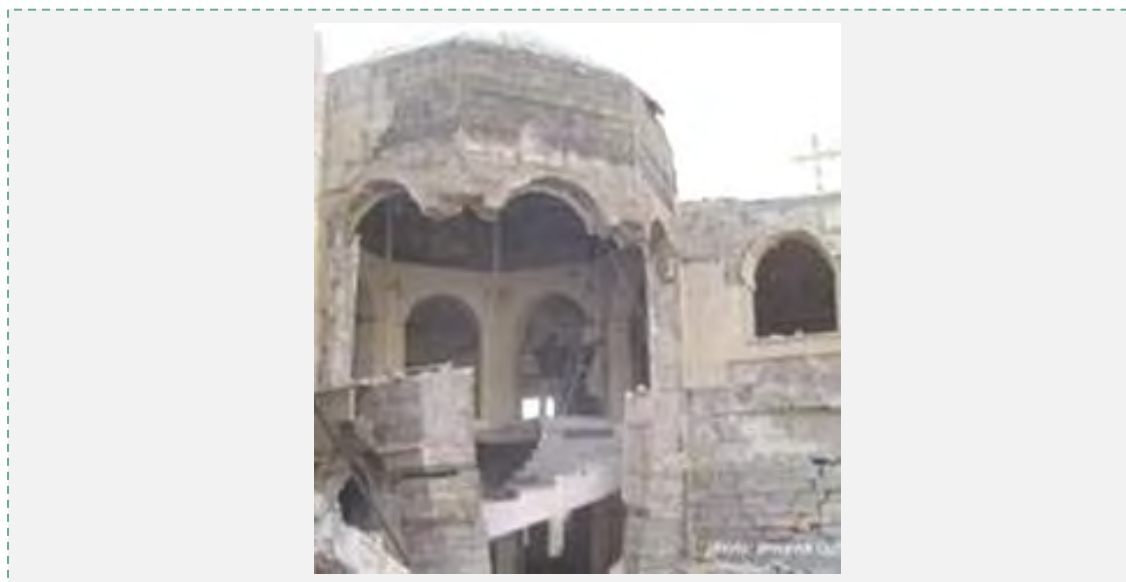
A Mosul church vandalized after ISIS occupation the city in June 2014. The media claimed that it had been demolished by IEDs (Abnar.ir).
