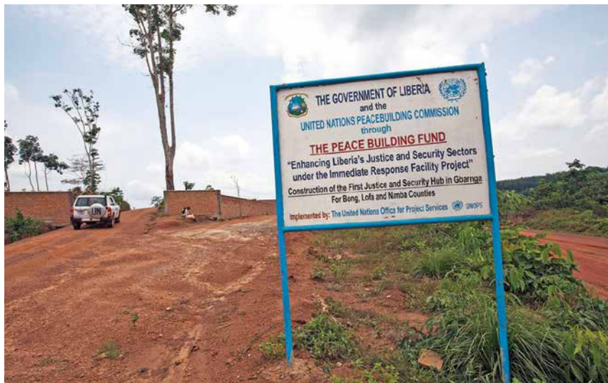
A sign at the entrance to the Gbarnga Justice and Peace Hub construction site in Gbarnga, Bong County, Liberia. Inaugurated in 2013 and featuring courts, barracks and training centres for security agencies, the $3.7 million Hub was paid for by the Peacebuilding Fund and built by the United Nations Office for Project Services. 13 APRIL 2012/UN PHOTO/STATON WINTER
