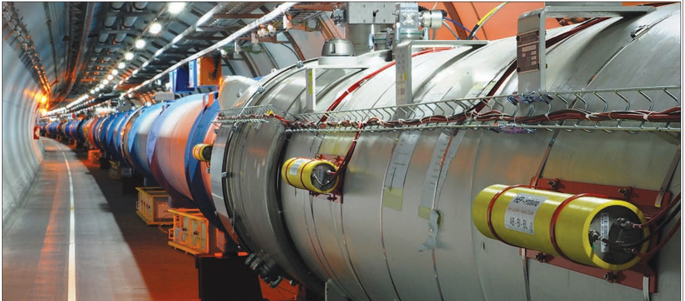
Beam-loss monitoring ionization chambers (the yellow tubes on the red supports) mounted on an LHC quadrupole magnet.
