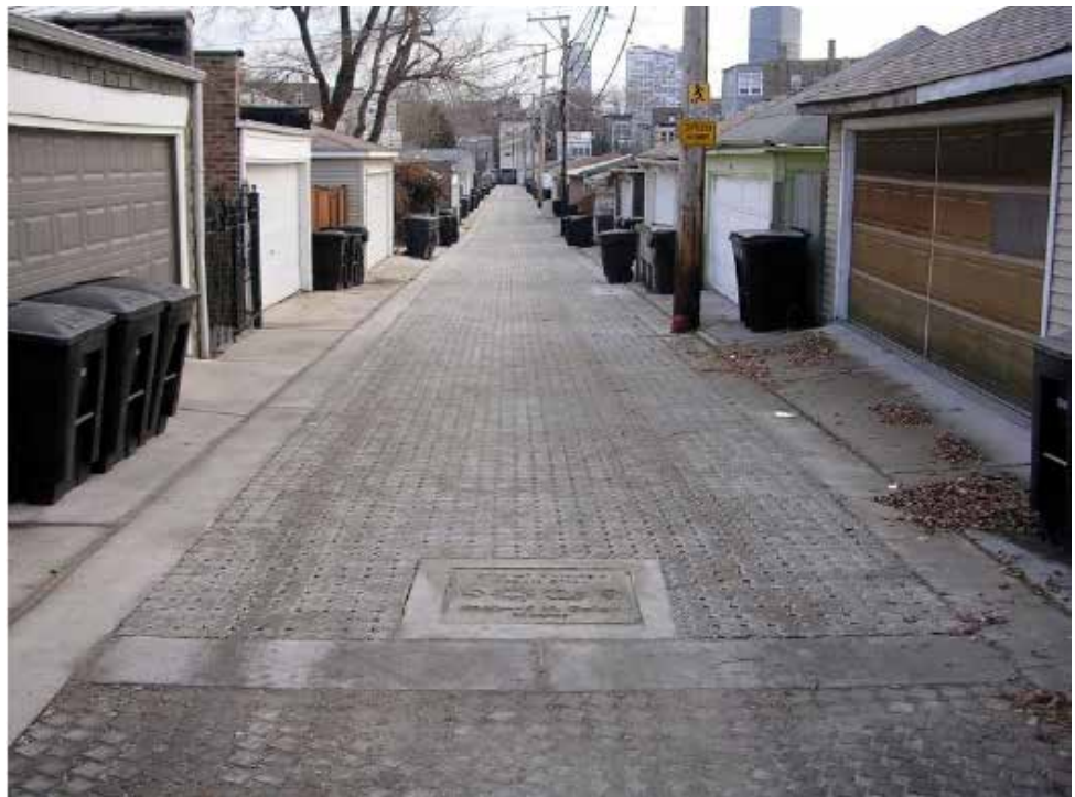
Figure 9.7: Permeable pavement in an alley in Chicago, IL.
