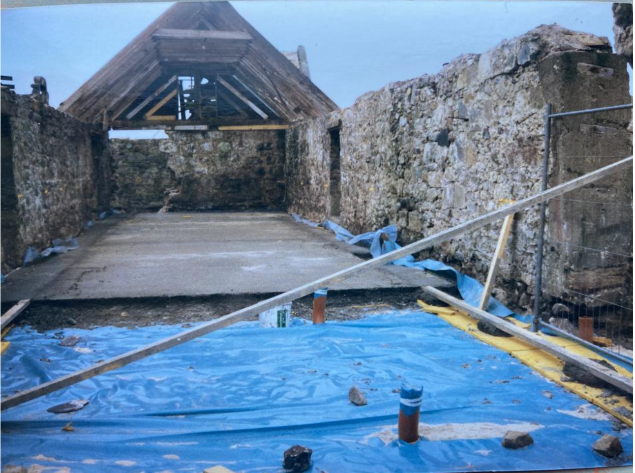
Image 6 – View of 1999 replacement concrete floor works indicating depth of concrete slab and presence of DPM
