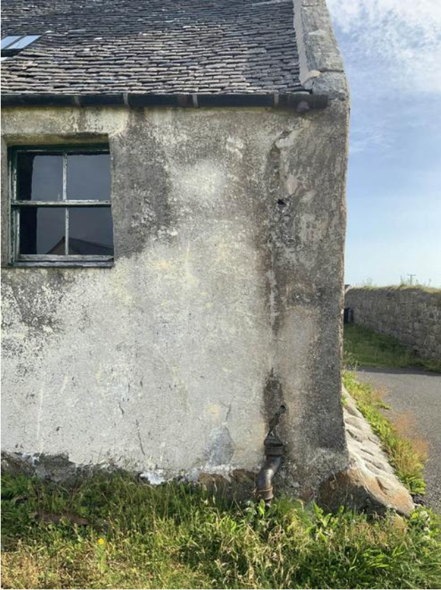
Image 10 – Example of missing rainwater goods
