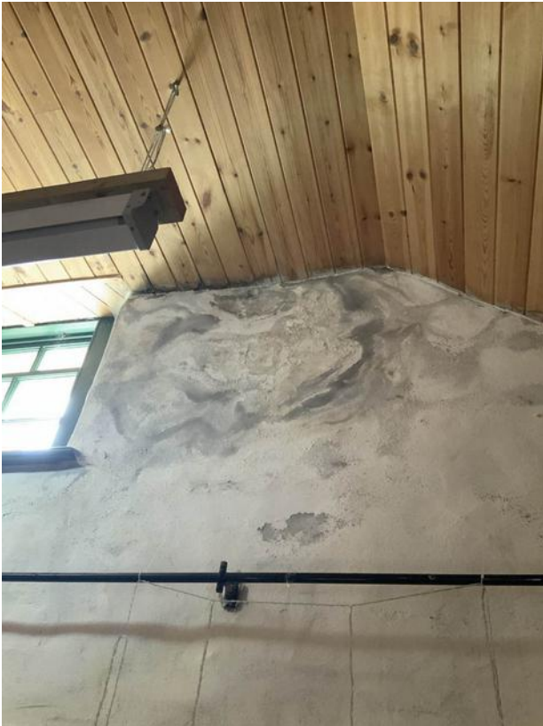
Image 17 – Example of area of damp
