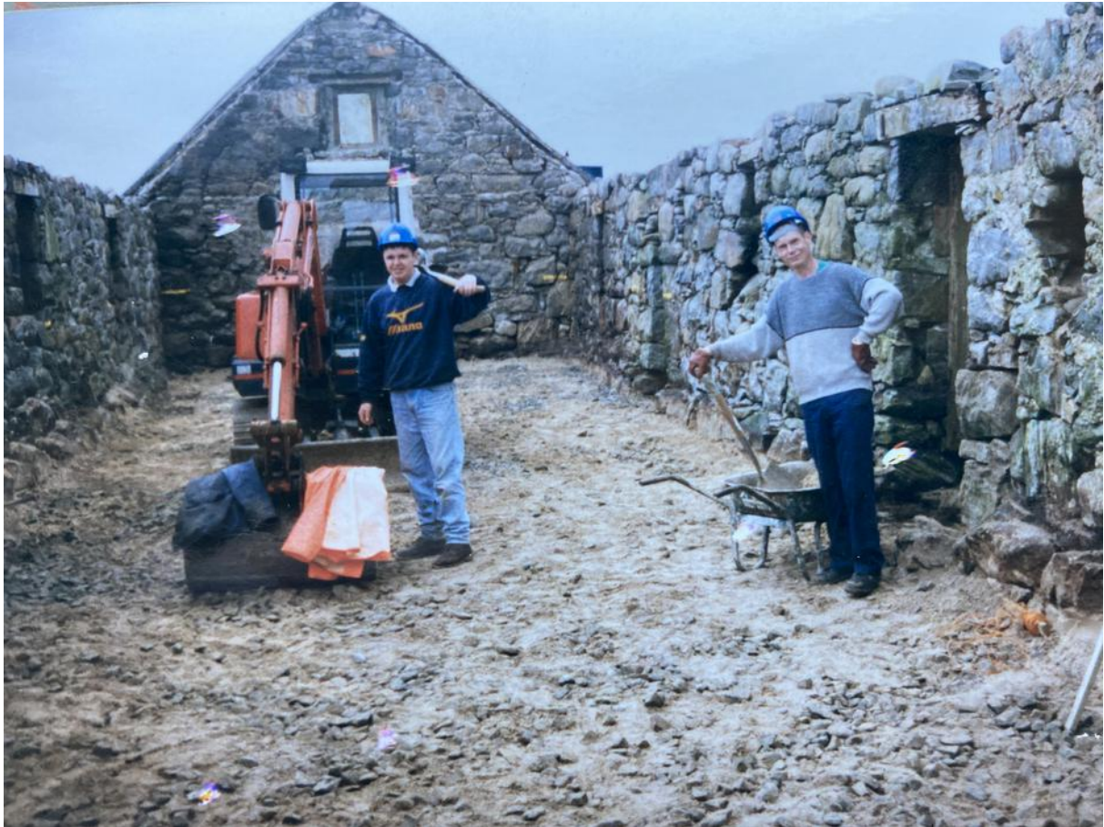
Image 5a and 5b – View of 1999 replacement concrete floor works indicating depth of excavations and existing drainage, North Wing – To become Still Room
