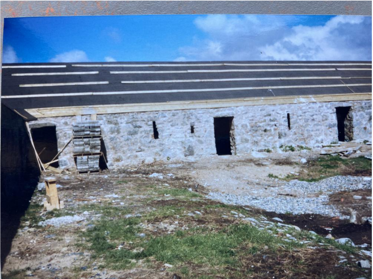
Image 16 – Image showing finished openings and use of Type 1F (non Breathable) Roofing Felt (1999 Works)
