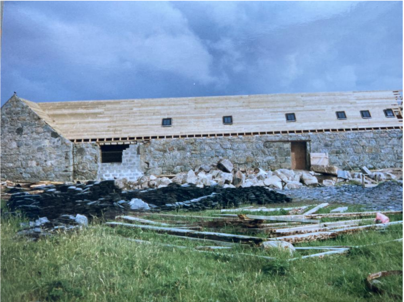
Image 15 - Area to Rear of Steadings showing replacement roof, blockwork to old cart opening, disturbed ground.(1999 Works)
