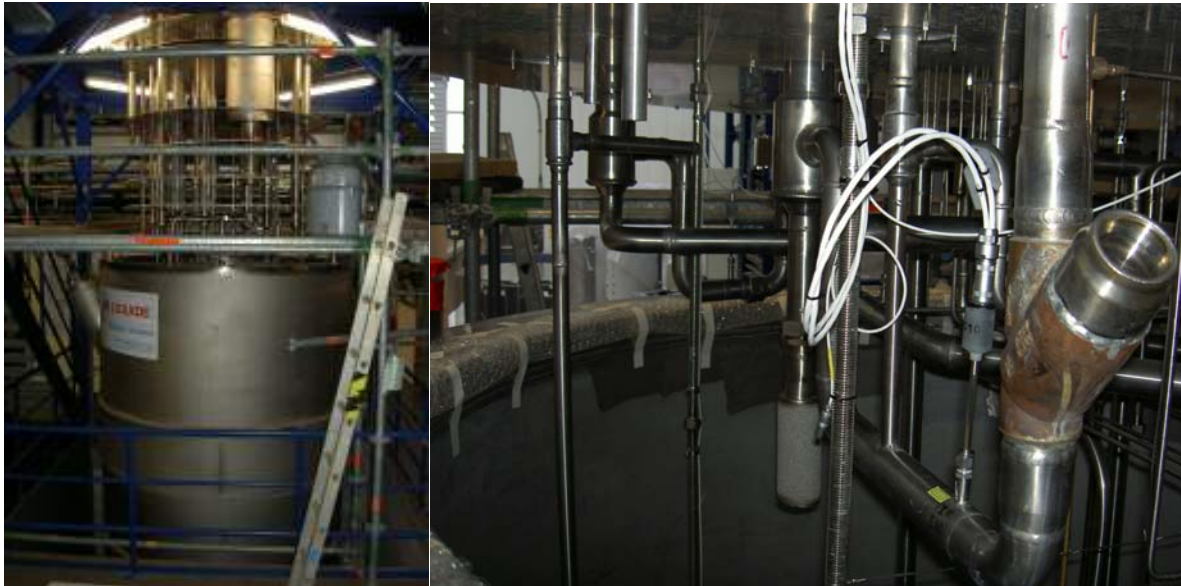
Fig. 1: Revision activities at the 5 K control cryostat of TIMO-2.
