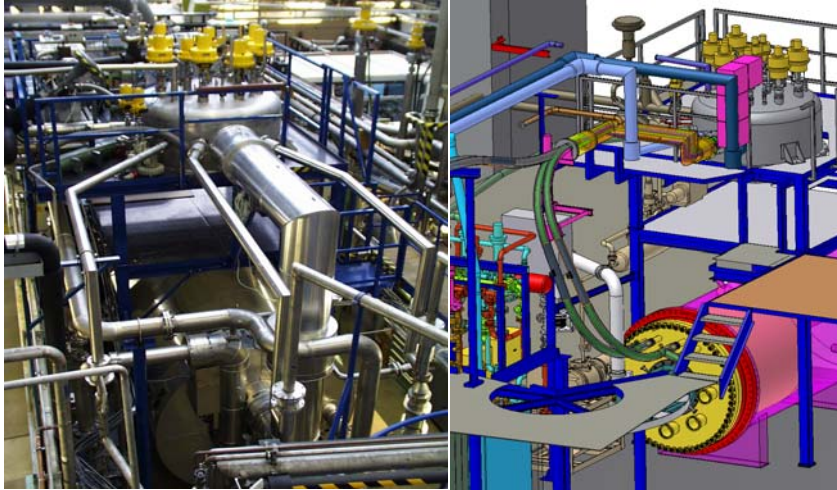
Fig. 4: Configuration of the old (left) and the new (right) cryo transfer line between the TIMO-2 valve box and test vessel flange.
