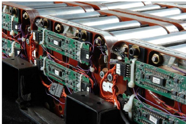
Fig. 5. Lead–acid battery and Li-ion pack.
