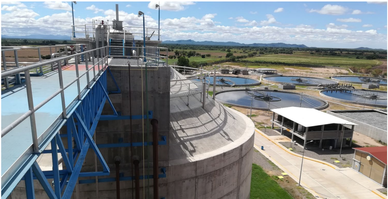
Figure 29. Anaerobic digester and secondary clarifiers in Hermosillo WWTP
