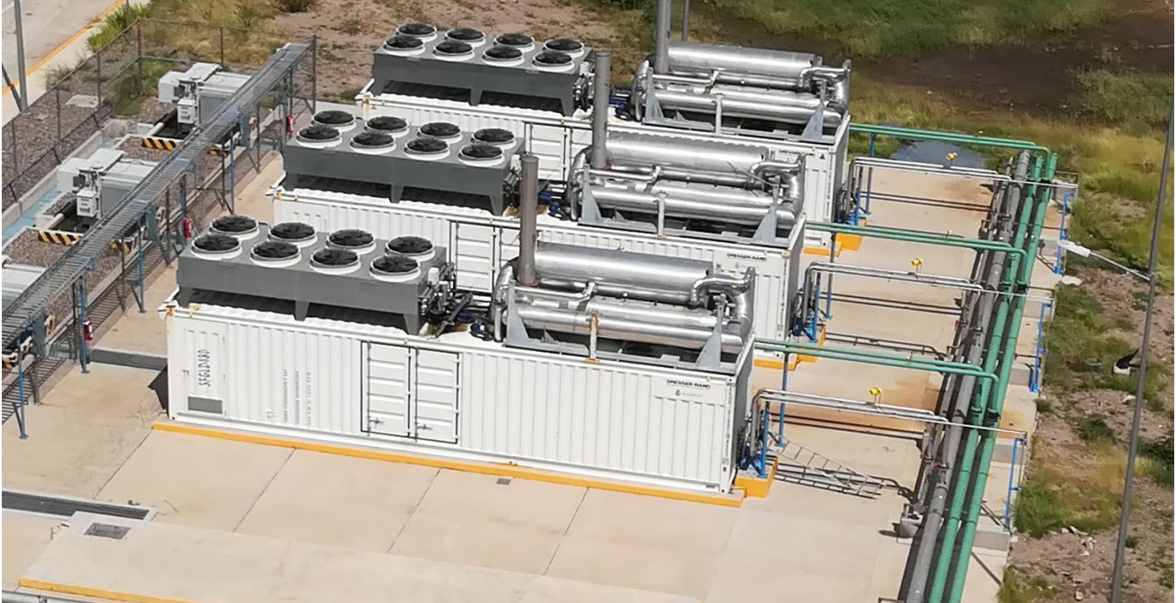
Figure 33. Three cogenerators (874kW) in Hermosillo WWTP (new but not operating). A basement for a fourth cogenerator is already built.
