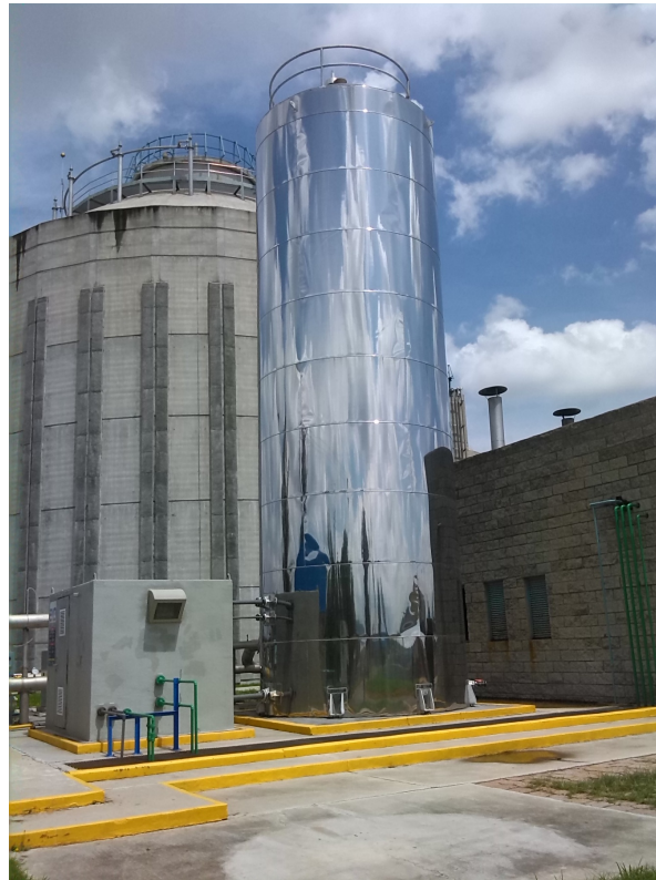
Figure 47. Biogas Clean installed in León WWTP (Courtesy: ECOSYS III/ FYPASA)
