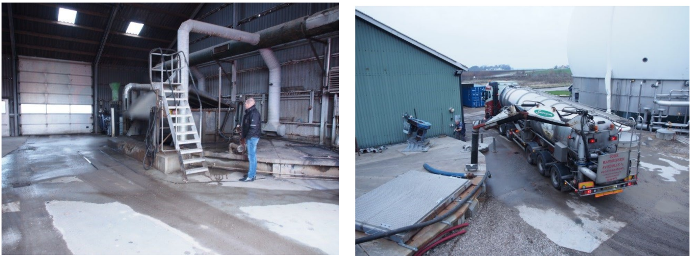
Figure 45. Example of a 600m 3 receiving tank underground at Hashøj biogas plant in Denmark (110 000tons/year). Trucks deliver under a covered in order to avoid smell (left) and pipes deliver feedstock outside into closed pipelines. (Courtesy: Bodil Harder/DEA)
