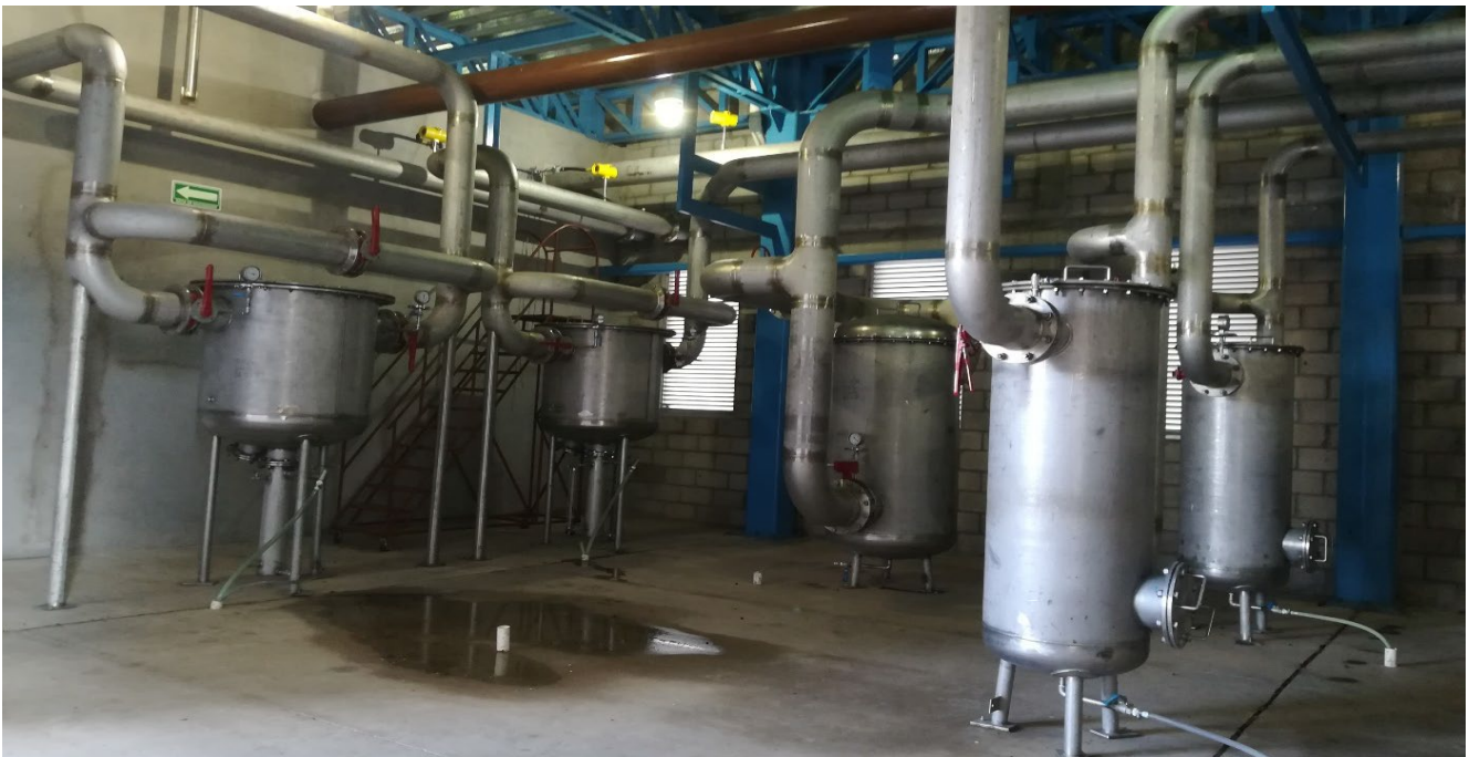
Figure 32. Condensate-sediment traps and filters for biogas
