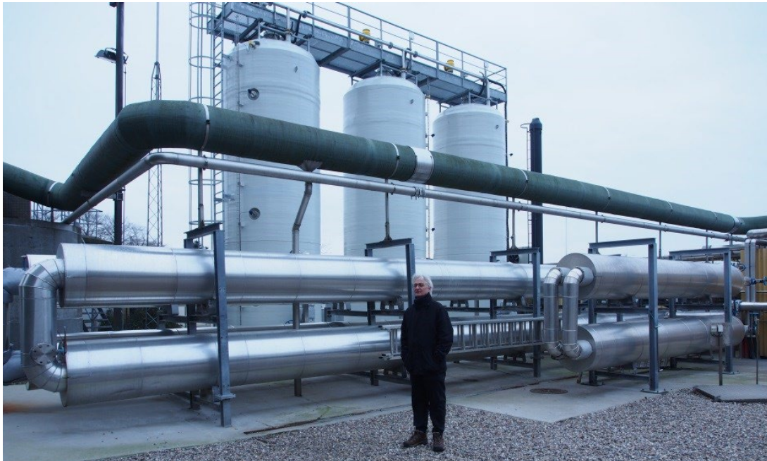
Figure 49. Example of three pasteurized tanks (back) and heat exchangers (front) at Hashøj biogas plant in Denmark (110 000tons/year). (Courtesy: Bodil Harder/DEA)
