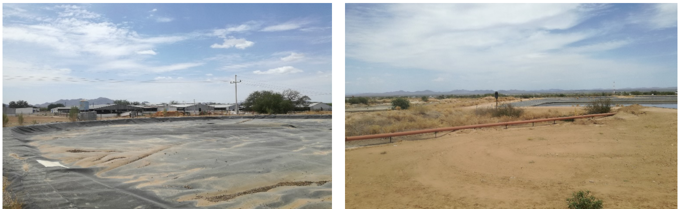
Figure 7. Covered anaerobic lagoon not in operation (left) and a not covered lagoon (right); no methane capture and use/burning and no proper treatment and reuse of water and nutrients.
