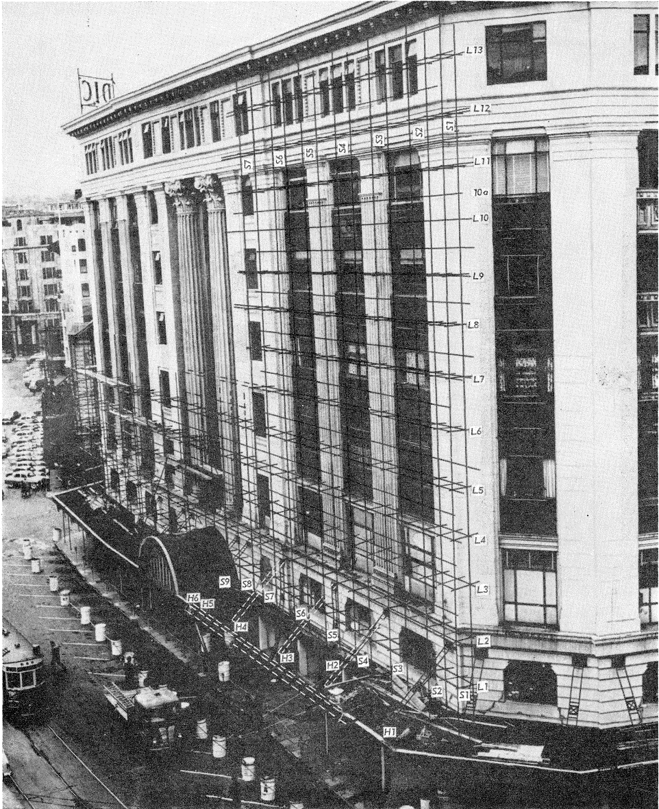
Prepared in the Ministry of Works District Office, Wellington. Scaffold as at time of failure.
