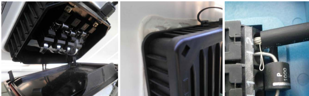
Fig. 6.1.3: Junction box failures: Left photo shows an open junction box in the field, the middle one a poorly bonded JB on the backsheet, and the right one a JB with poor wiring.
