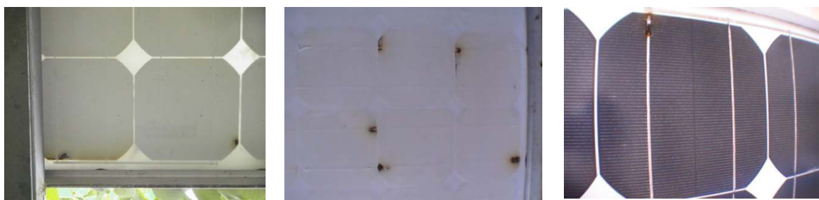
Fig. 6.2.22: Burn marks caused by open-circuit bypass diodes.
