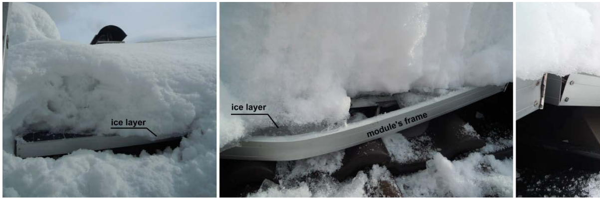
Figure 6.1.4: Damaged module frames after heavy snow load of 1.2 m, melted down to 35 cm, in winter 2012. Alpine location at 620 m a.s.l., tilt angle 25°. 60 cell modules with dimensions 1660 mm x 990 mm, 50 mm Al-frame. Left hand side: Ice layer slides over module's edge; Middle: Ice bends frame; Right: Failure of the corner screw joints [Leitner12].
