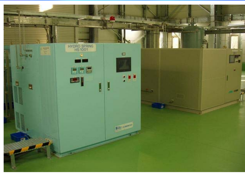
Left ; Hydrogen Generator( PEM Type ) : 1.0 Nm 3 /h, 20 N l/min Right; Hydrogen Storage Tank ( Metal Hydride Type ) : 10 Nm 3 /h, 1Nm 3 /h
