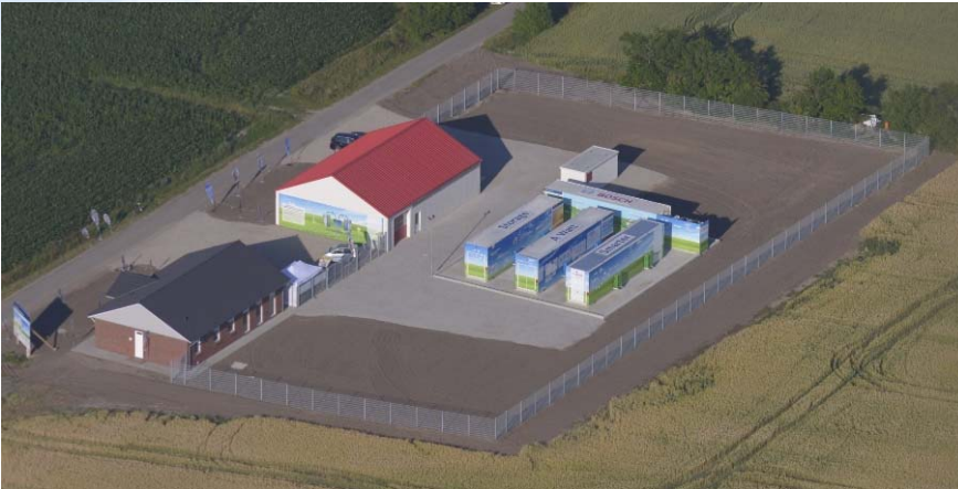
Braderup: 2 MWh li-ion battery + 1 Mwh vanadium redox flow battery
