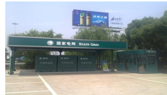
Charging/battery swap station in Jiaxing Service area
