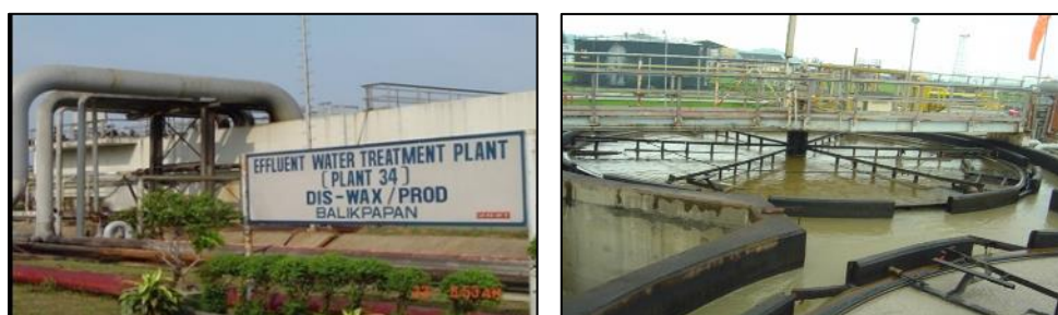
Figure 2.6 Existing effluent water treatment plant.
