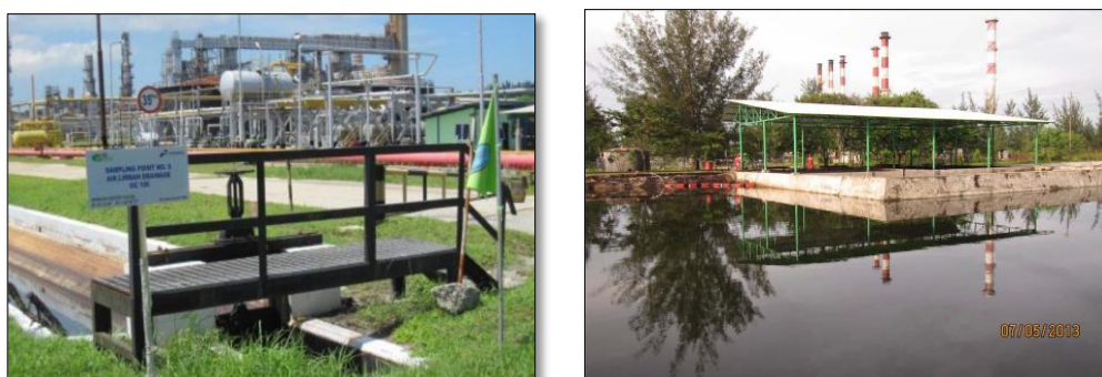
Figure 2.7 Oil catcher and sludge oil recovery system.
