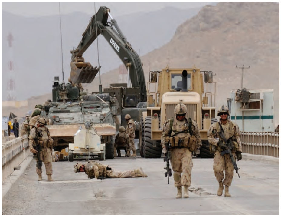
Canadian engineers repair bridge damaged by suicide car bomb in Kandahar, Afghanistan
