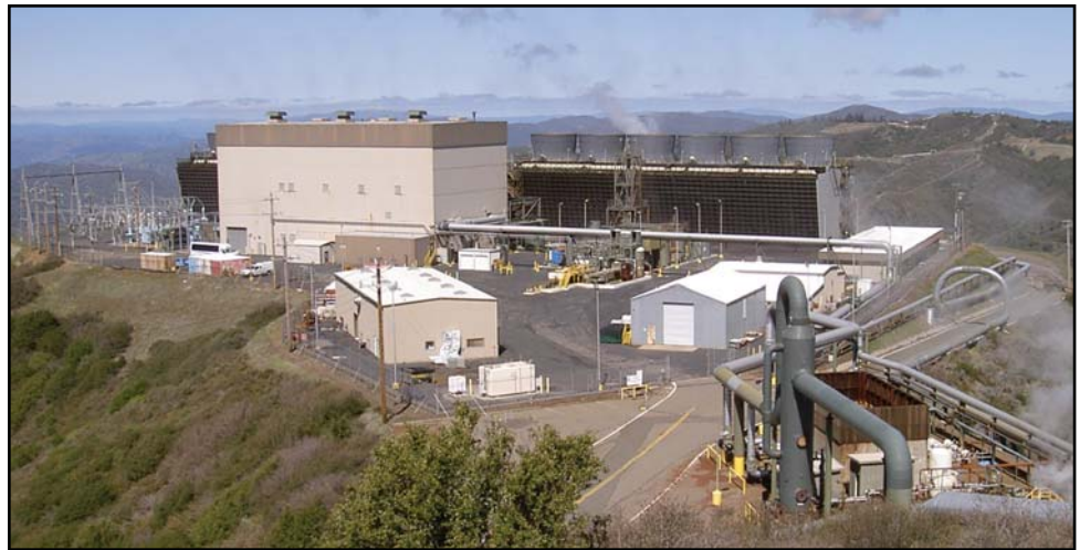
Figure 7.5: The Sonoma Calpine 3 power plant, one of 22 power plants at The Geysers field in the Mayacamas Mountains of Sonoma County, northern California.
