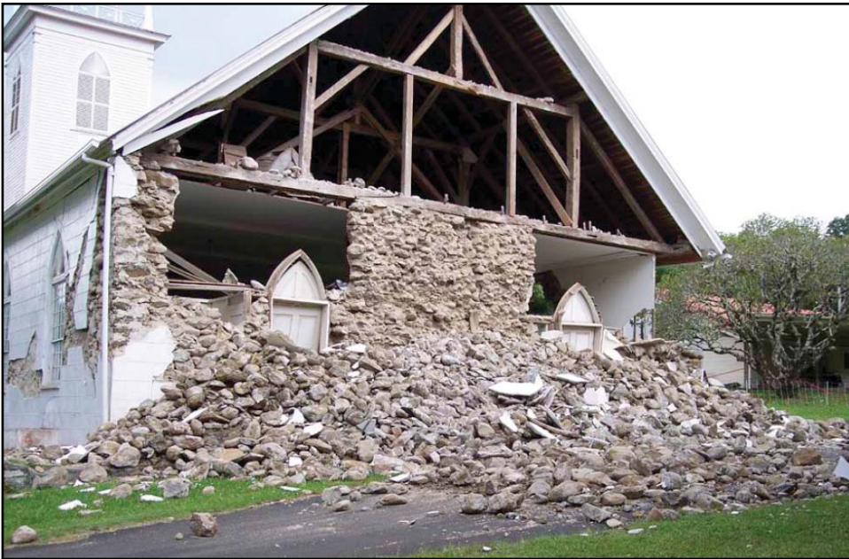
Figure 10.24: Kalāhikiola Church, Kapa'au, Hawai'i Island, 41 kilometers (25 miles) from the epicenter of the 2006 Kīholo (M6.7) earthquake.
