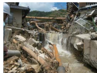
Photo 1. Exposed Distribution Mains after 2014 Landslides in Hiroshima
