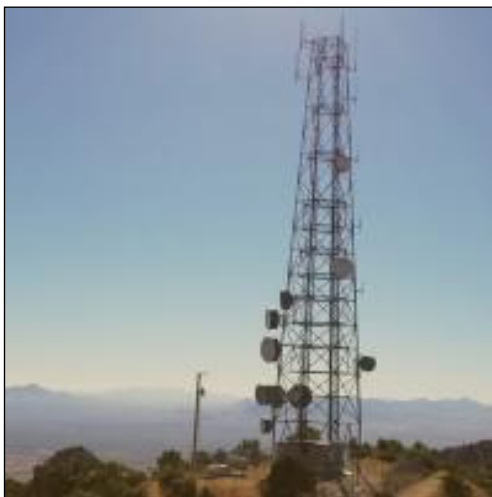
Communications Tower, BLM photo
