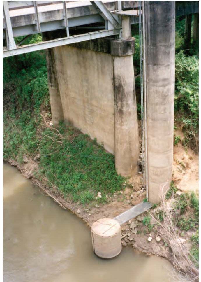
Figure 8. In-bank stilling well and silt trap.
