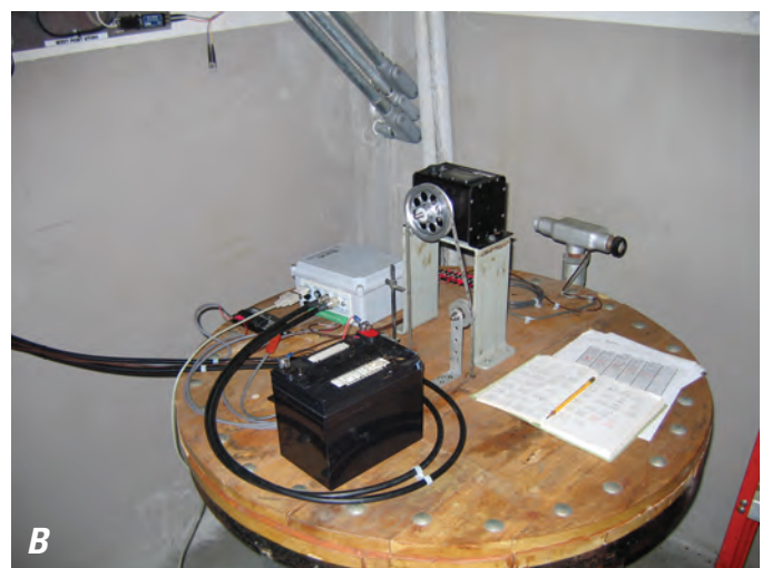
Figure 47. A, Typical installation of float-tape gage and B, electronic shaft encoder and electronic data logger (EDL).
