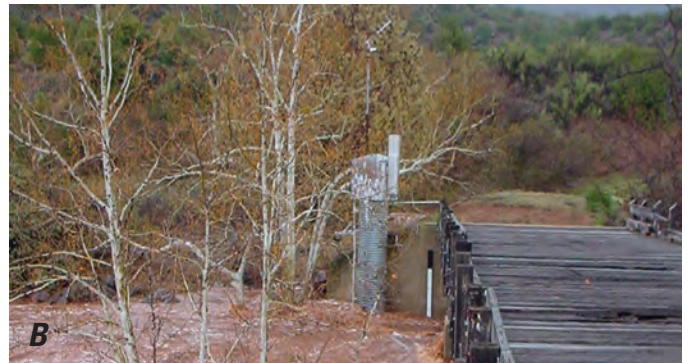
Figure 5. A, Steel pipe stilling well and B, shelter attached to bridge abutment.
