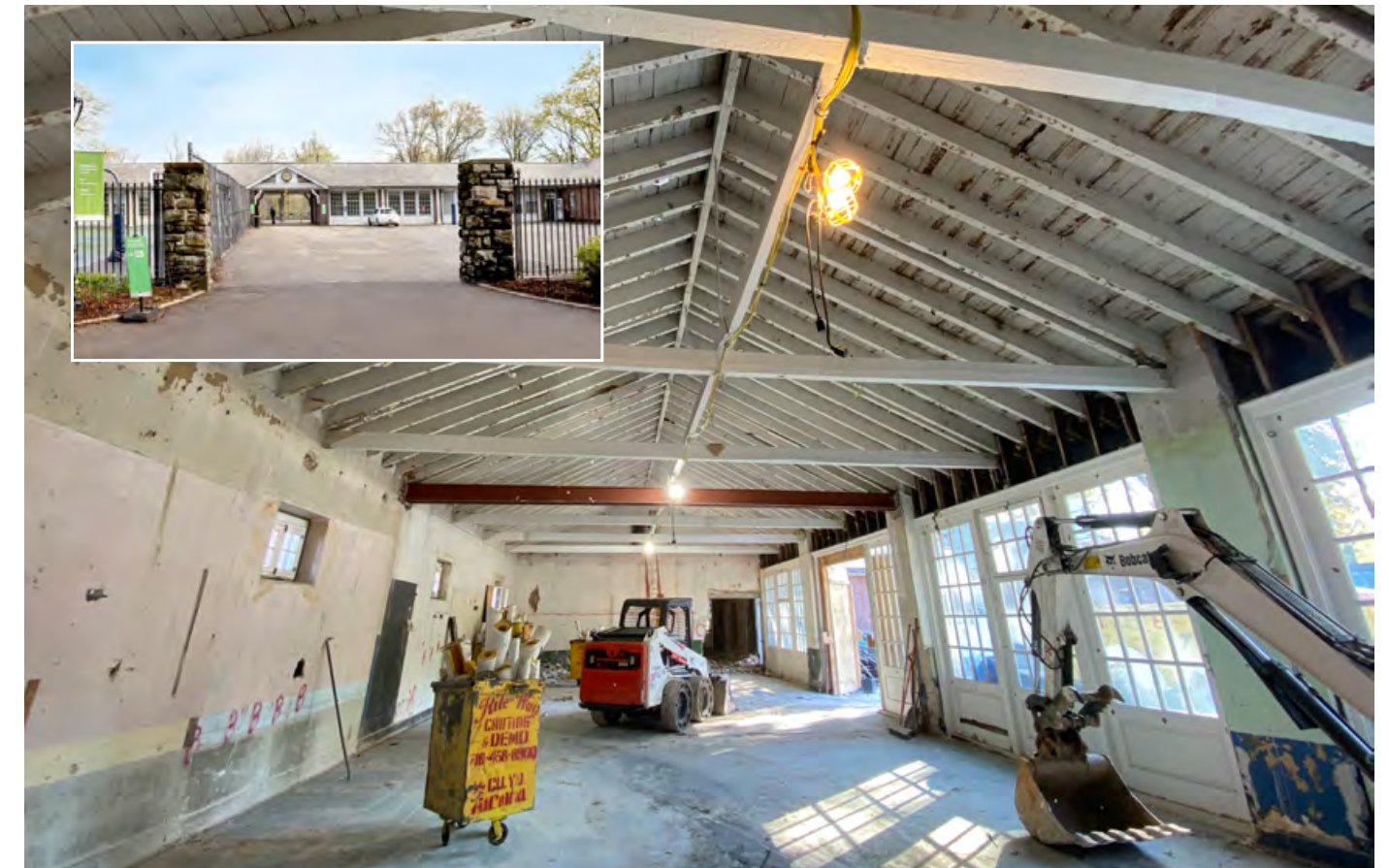
Interior demolition at North Meadow Center; Inset: Building exterior prior to start of construction
