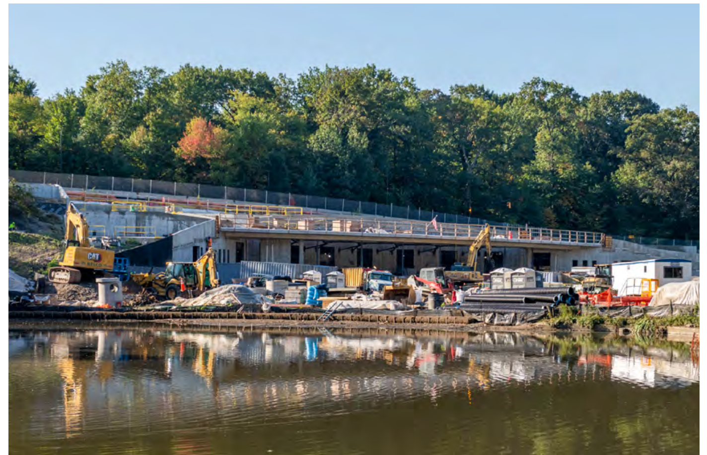
Above: Ongoing construction at the Harlem Meer Center; Opposite page: The newly renovated Chess & Checkers House and Kinderberg rustic structure
