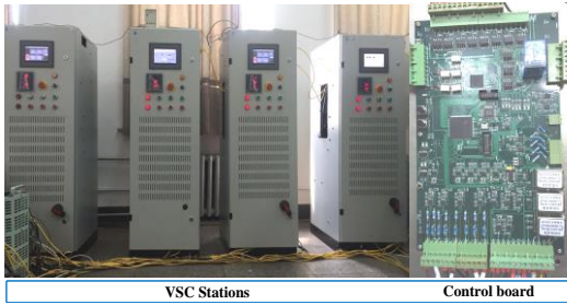
Fig. 15: VSC converters of experimental platform and main driver board of the power converters (right).
