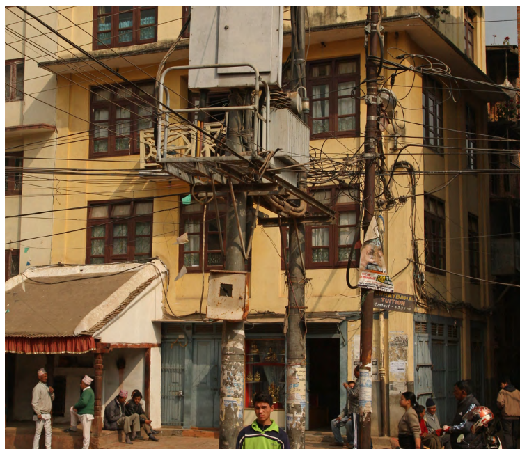
Electrical lines, Kathmandu, Nepal. © Simone D. McCourtie | World Bank.
