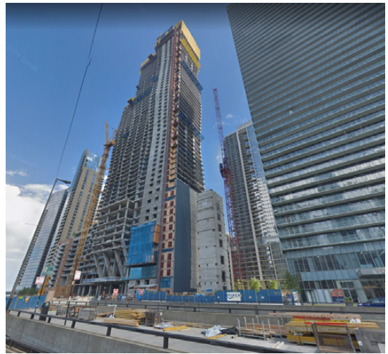
Construction of Vista Tower and other high-rise office and residential buildings, in accordance with the Central Area Action Plan | Source: © Google Maps, Street view of Vista Tower Construction | https://tinyurl.com/yazbl7ff Waterfront
