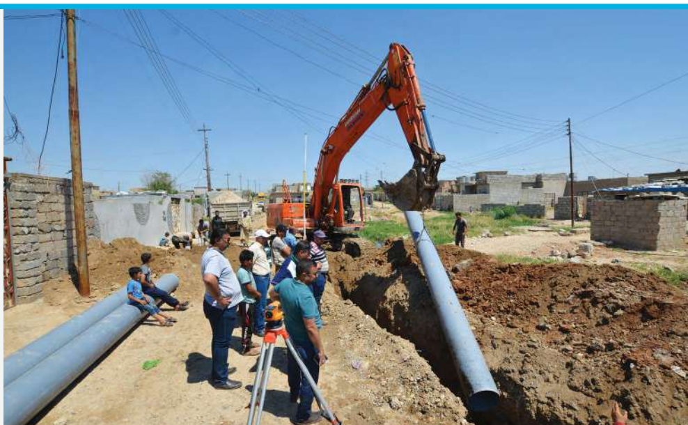
Instalment of drainage and potable water network at Hay Tanak, West Mosul, Iraq
