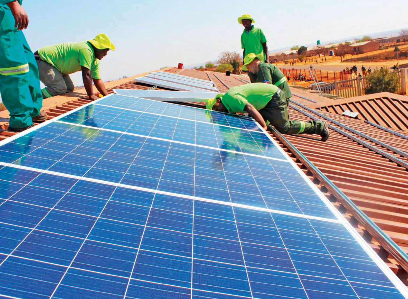
Solar panels installed through project funds on a community building in Steve Tshwete Local Municipality, South Africa
