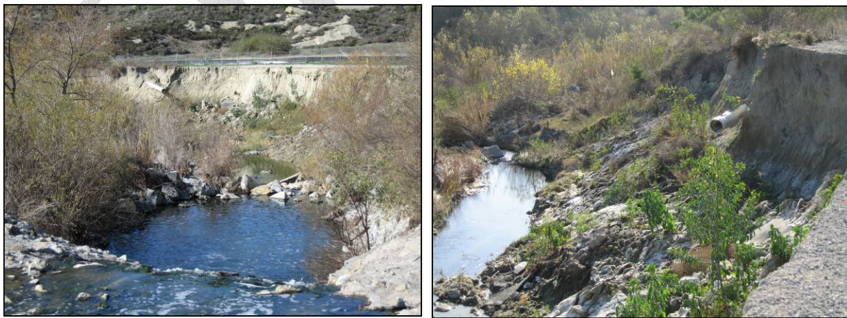
Channel erosion downstream of ACWHEP
