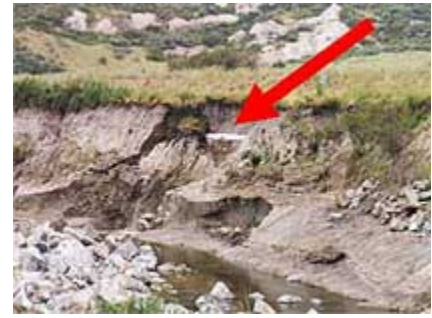
Exposed utility pipeline in Aliso-Wood Canyon Regional Park.
