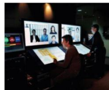
Remote control room
