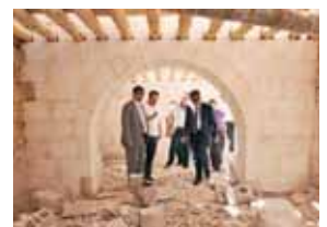
Old, historic structures throughout the Şehitkamil Municipality are being lovingly repaired and restored.
