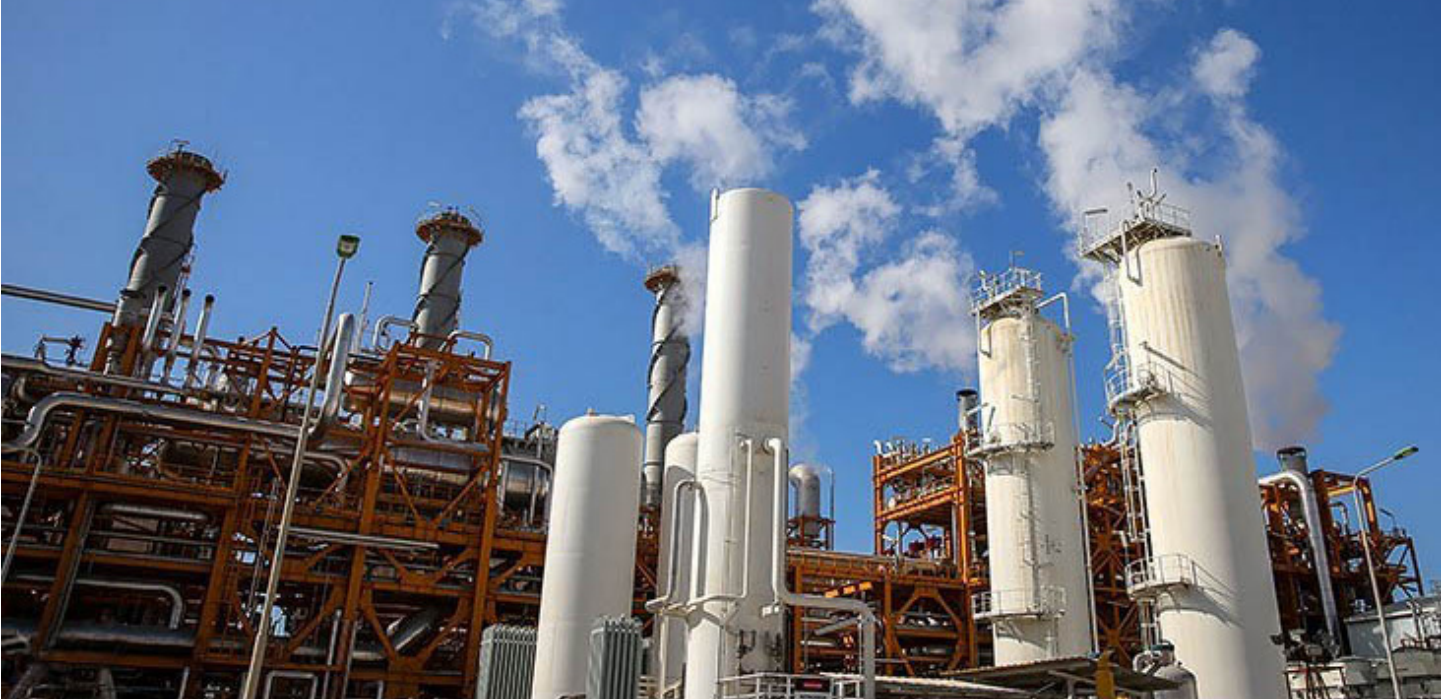
South Pars Onshore Facilities near Asaluyeh City, December 11, 2013. Photo: Wikimedia Commons, Hamed Malekpour
