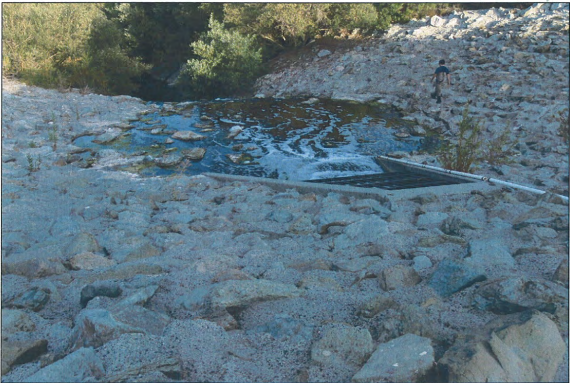
H) Small, shallow pool at downstream end of culvert beneath the road crossing, facing downstream.
