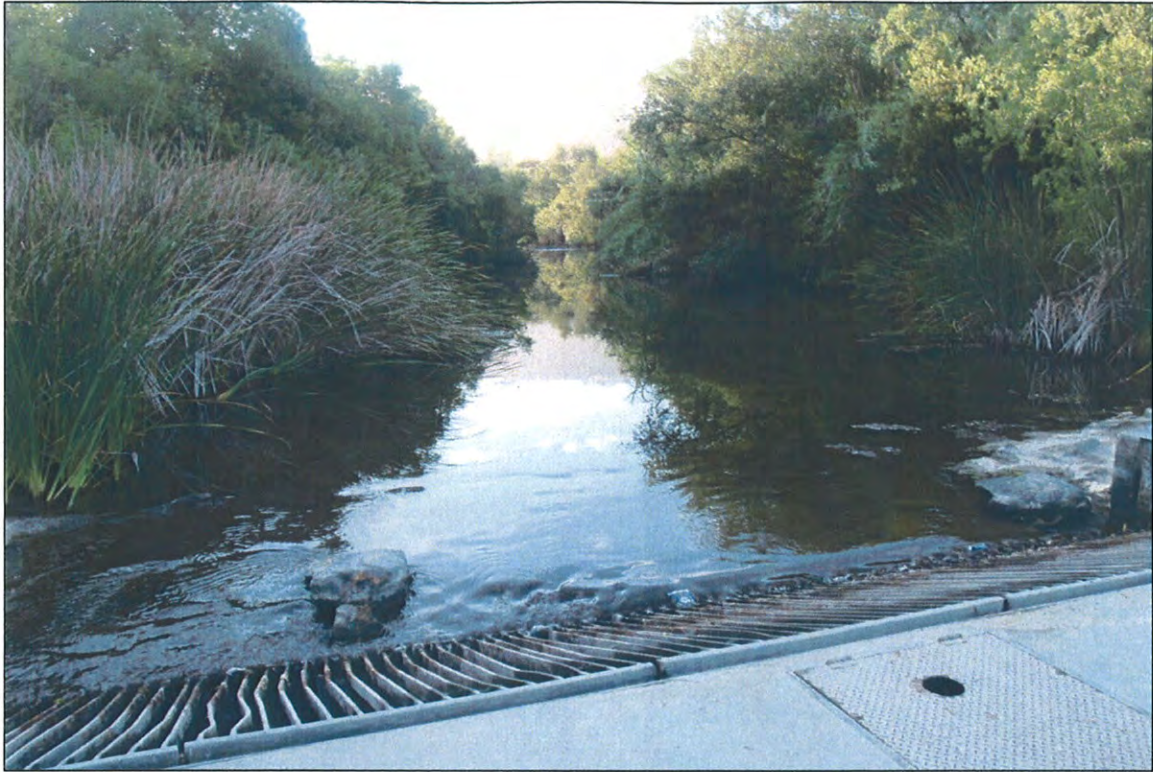
G) Bar racks on the upstream end of the culvert located within the concrete dam/road crossing, facing upstream.
