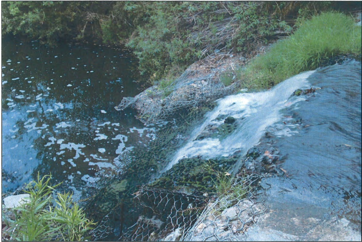
K) Drop structure (5 to 6 ft high) located at the upstream survey boundary, Alicia Parkway overcrossing.
