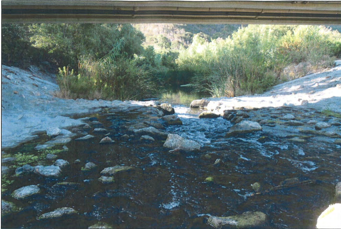
A) Concrete covered riprap channel beneath the bridge leading to the Coastal Treatment Plant, facing downstream.
