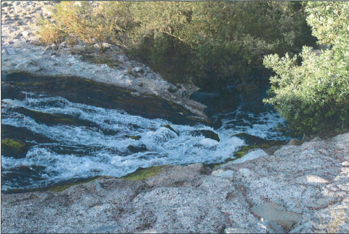
I) Steep gunited spillway (8.5-m long with 30 percent gradient) below the small pool immediately downstream of the culvert opening.
