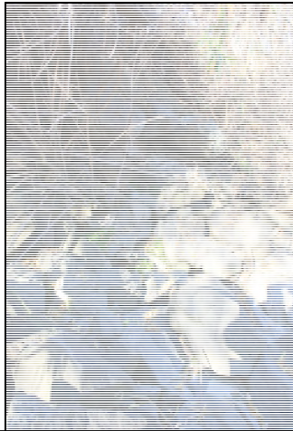
34 Oversteep / Undercut Riprap (looking u/s) Emergency rock placement? Near-vertical rock on bank. Stable toe. Geotechnically stable bank?
