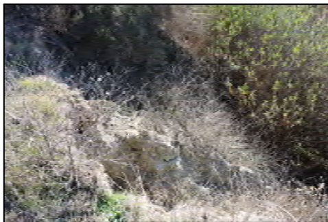
7 Impingement & Concentrated Runoff
