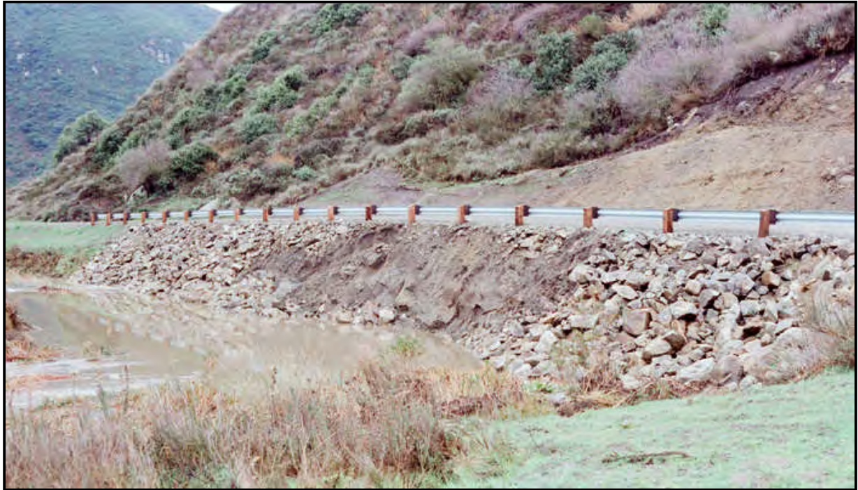
Figure 1-4. Emergency Repair of West (right) Bank of Aliso Creek (photo courtesy of SOCWA, appears to be near RM 1.85)
