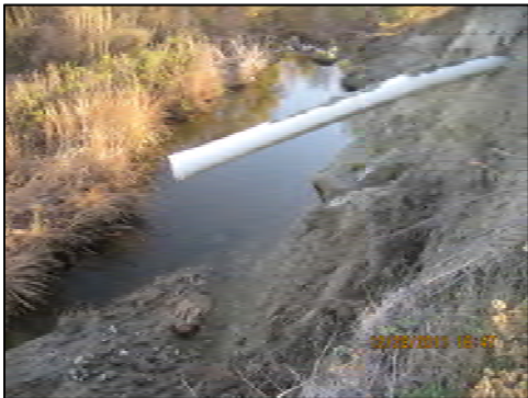
15 Flow Impingement, Slumping (looking d/s) Direct impingement of flood flows; slumped material at toe.
