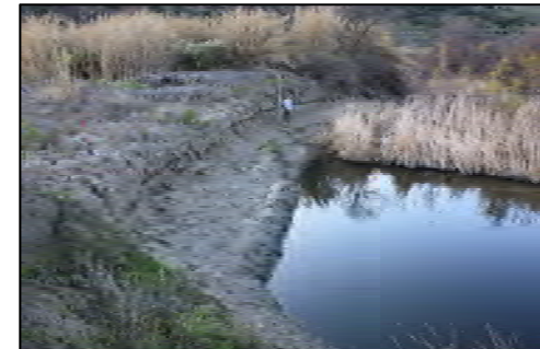
32 Probable Future Incision (looking d/s toward bend) Active erosion in chute (red shovel). Bend persists since pre-1930. Clay in toe of bank reduces rate of erosion/migration.
