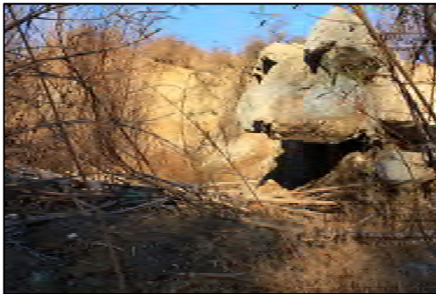
14 Undercut Riprap Threatening ACWHEP diversion structure.
