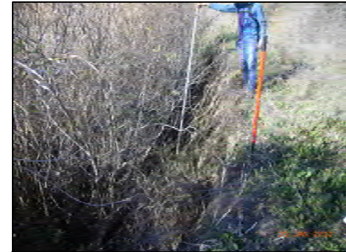
2 Upper Bank Geotechnical Instability
