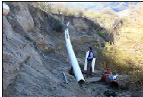
21 Leakage along Abandoned Pipe, Slumping, Impingement
