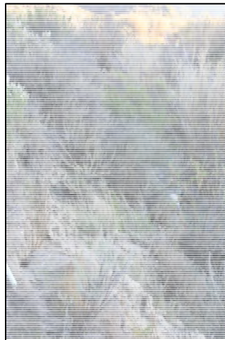
30 Flow Impingement (looking d/s) Flood flows in Aliso Creek erode bank material upstream of existing riprap revetment.
