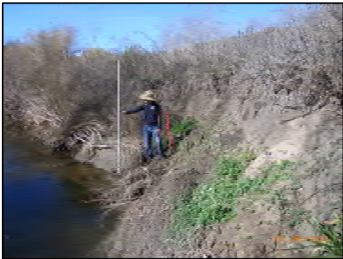
12 Flow Impingement (looking d/s) Outside bend upstream of ACWHEP backwater influence, unstable bank.
