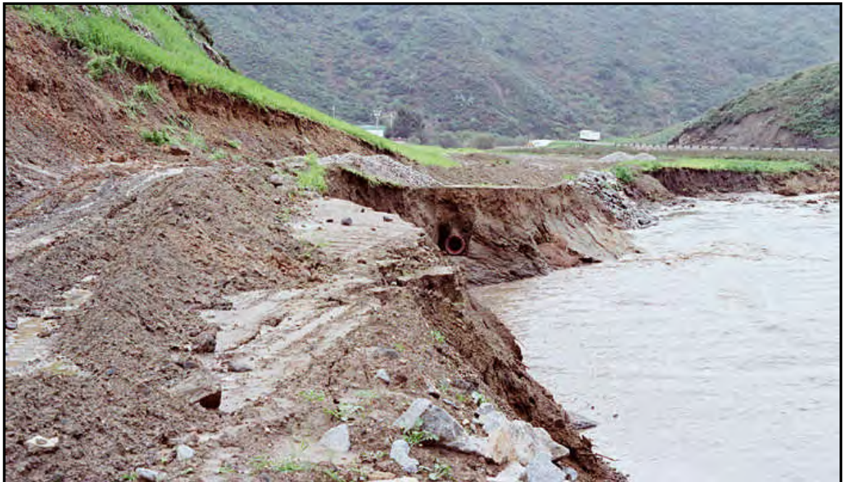
Figure 1-3. East (left) Bank Erosion along Aliso Creek Showing Undermined MNWD Pipeline (photo courtesy of SOCWA, appears to be near RM 1.60)
