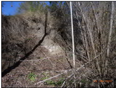
10 Upper Bank Instability (looking u/s) Close proximity to alignment. Lower bank stable and vegetated, scarp along upper bank.
