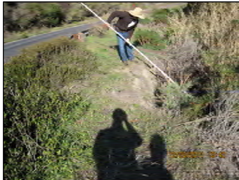
31 Flow Impingement, Narrow Setback Active flow impingement above elevation of riprap revetment along bank. Narrow setback. Also concentrated runoff down the bank.
