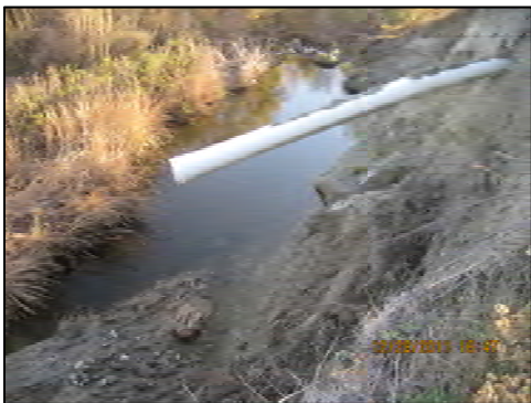
15 Flow Impingement, Slumping (looking d/s) Direct impingement of flood flows; slumped material at toe.
