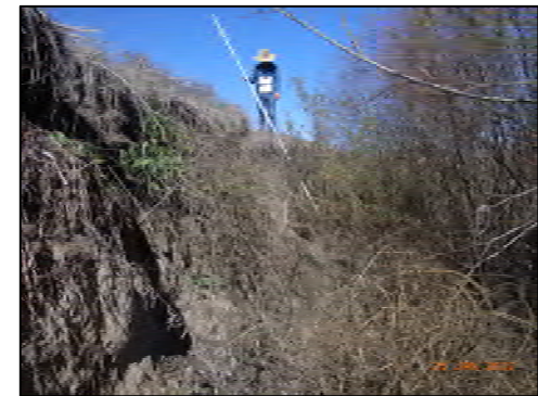
8 Upper Bank Geotechnical Instability (looking u/s) Close proximity to pipe alignment, further widening as upper bank stabilizes.
