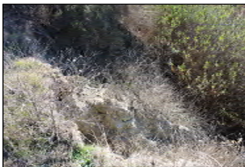
7 Impingement & Concentrated Runoff (Riverward view) Fluvial energy cutting into toe of alluvial fan; concentrated upland runoff contributes to bank failure. Steep high bank actively failing.
