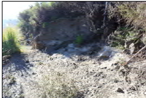
33 Oversteep Bank, Narrow Setback (looking d/s) Potential for continued fluvial erosion. Bank not geotechnically stable. Top of unstable bank within 15 feet of AMWA Road.
