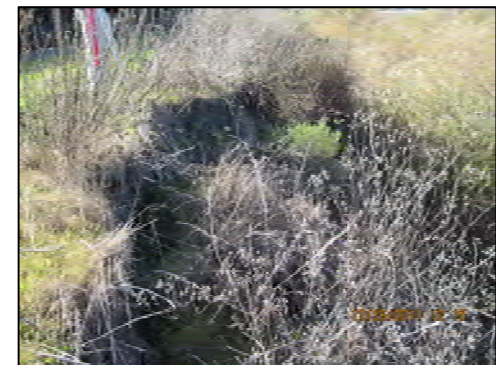
5 Slumping (looking d/s) No woody vegetation at toe to hold failed material. No room to lay back slope.
