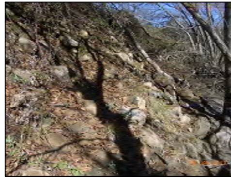
9 Impingement, Weathered Riprap (looking u/s) Riprap revetment to protect against impingement is breaking down.
