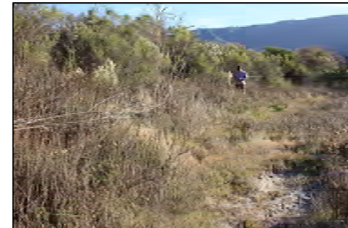
29 Stable Bank Downstream view of left bank, 2.5H:1V bank slope. Woody shrubs established across bank, stable toe along high flow chute.
