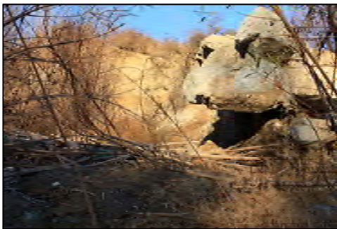
14 Undercut Riprap Threatening ACWHEP diversion structure.
