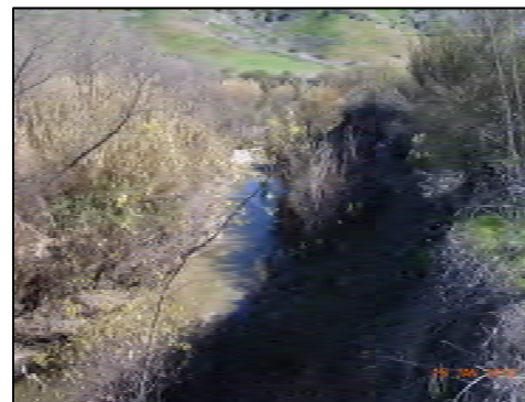
6 Upper Bank Geotechnical Instability (looking d/s) 30-ft high bank, nearly vertical. Close proximity to AMWA Road.
