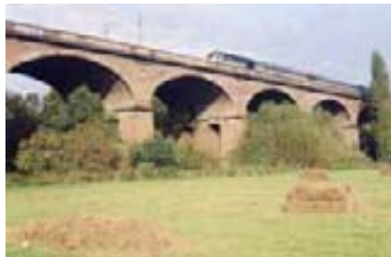
The 275-metre long Wharncliffe Viaduct still carries London-Bristol trains at an elevation of almost 20 metres across the Brent Valley in West London.
