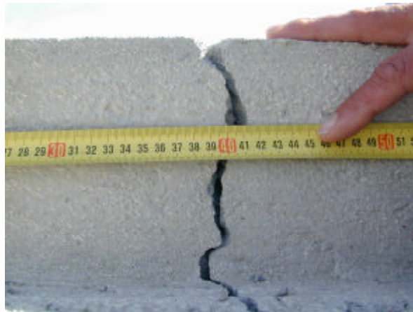
Figure I-20 : Width of a lean concrete crack.
