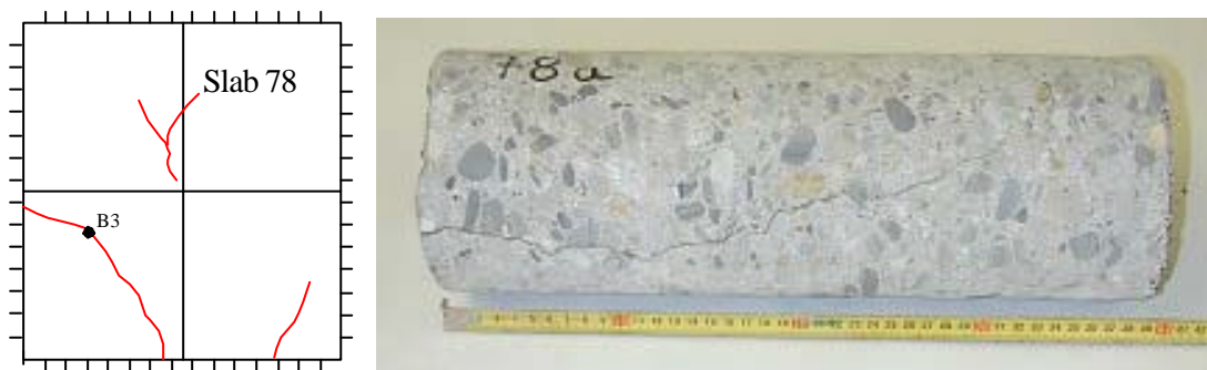
Figure IV-38 : Slab 78 – borehole b3 – Partial top to bottom crack.
