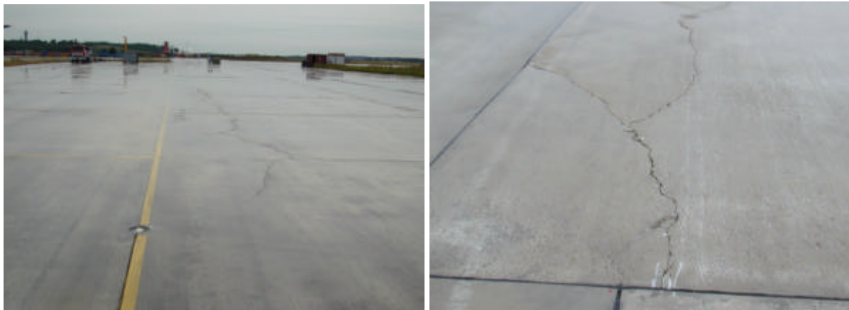
Figure IV-31 : (a) Example of longitudinal crack – (b) Example of corner cracks.
