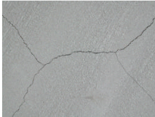
Figure I-18 : Cracking of the lean concrete.
