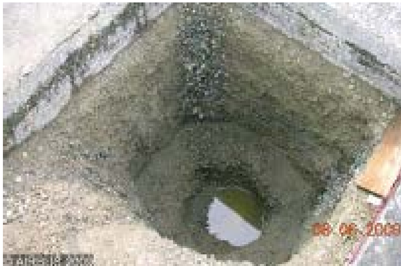
Figure 17 : Water contamination under the pavement
