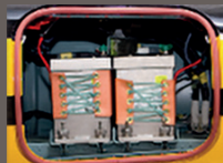
Second battery installation
